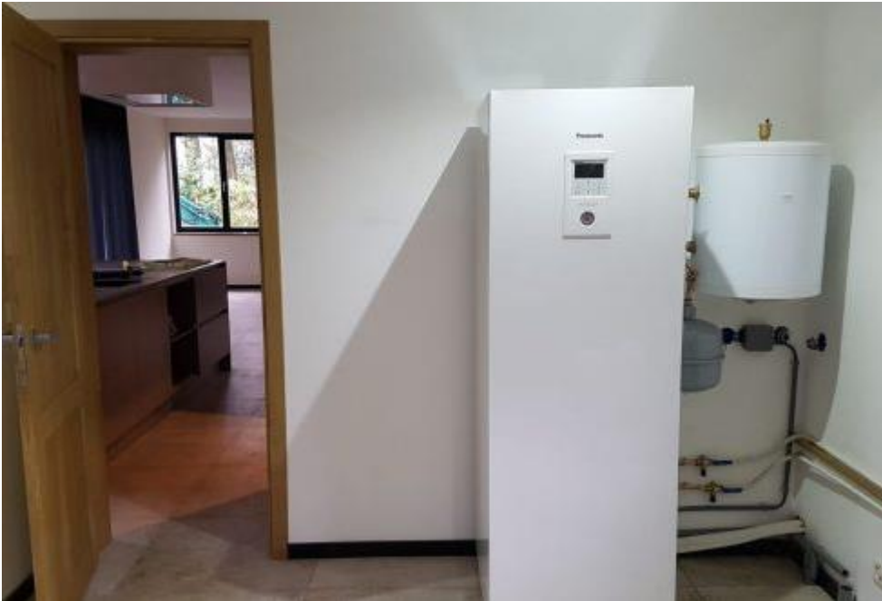
Binnenunit + warmwater boiler
